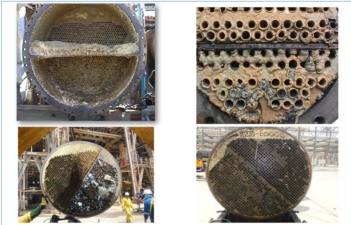
Figure 3 Tubeside fouling photos with plugging of tube holes
