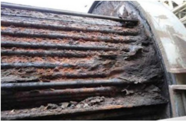
Fouling at vapor entry section of tube bundle
