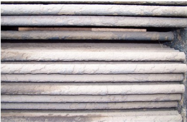
Fouling generally throughout tube bundle
