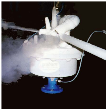
Liquid-nitrogen cooled, methylene chloride vent condenser cooling to -60 degrees F for 95% reclamation
