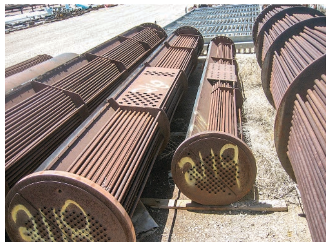
FIG. 6. A maintenance yard filled with failed bundles.
