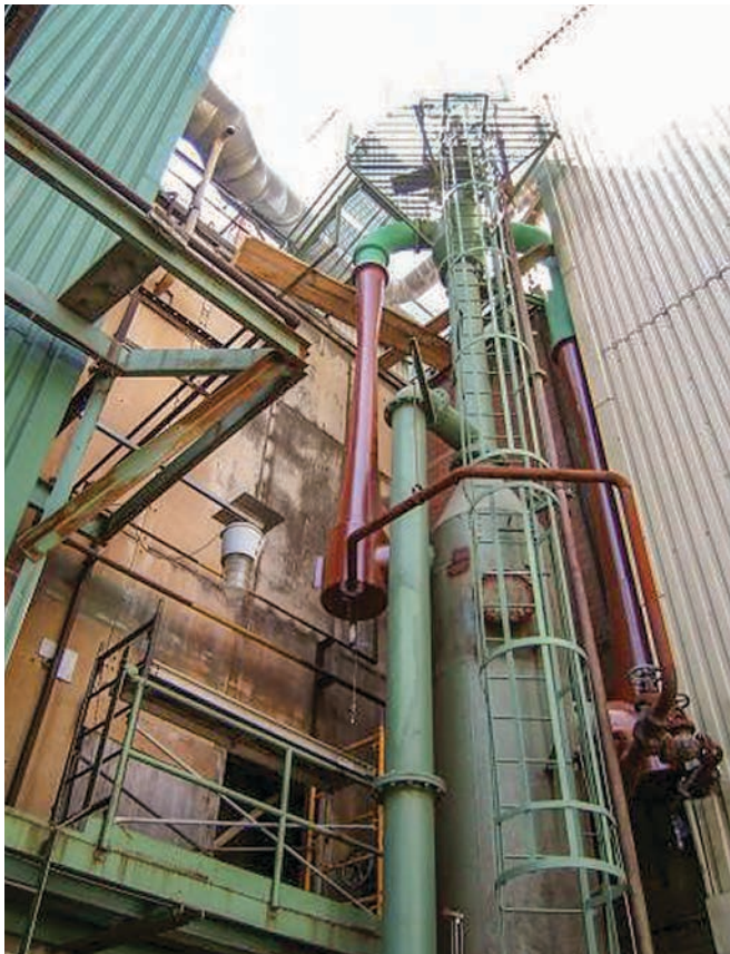
FIG. 5. OEM replacement ejectors on an SVRU.
