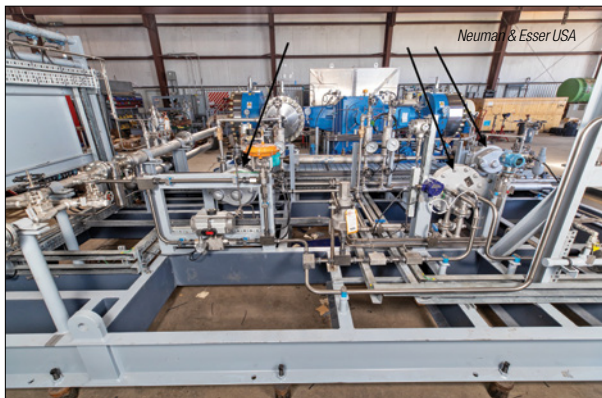
FIGURE 2. Three spiral-tube heat exchangers are shown here (arrows) within a Neuman & Esser hydrogen diaphragm-compressor package
