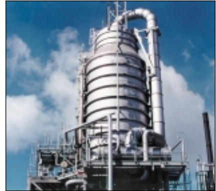
Flasher process vacuum condenser with piping from the process vessel to condenser.
