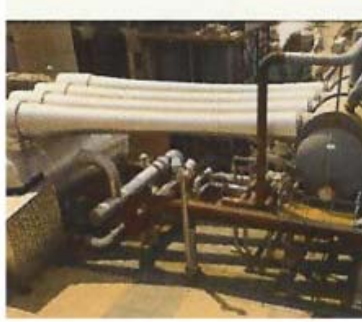
Vacuum refrigeration systems
